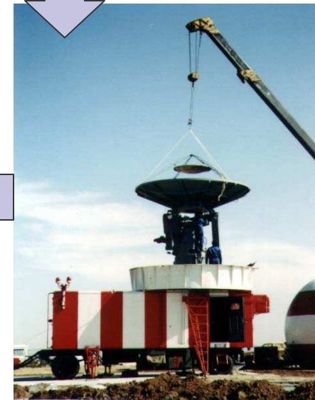
Radar Antenna Assembly
